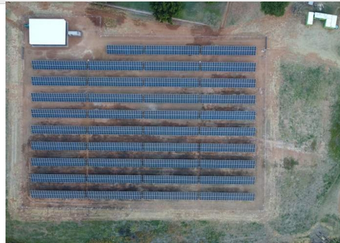
↑ 1,1 MW Ground mounted Installation
